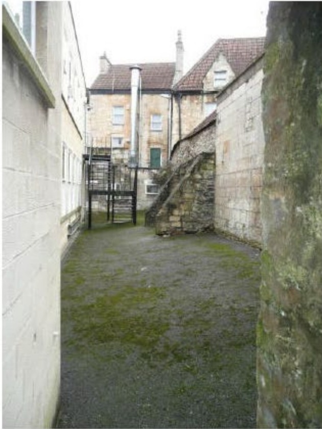
View 1- 4m high retaining wall on rear boundary to the Vintners ( see SK/120 )
